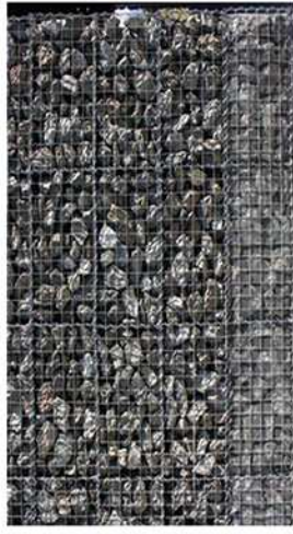
GABION HEDGE IN UNDERCROFT ARCH - OFFERS OPPORTUNITIES FOR SIGNAGE AND PARKING RESTRICTIONS
